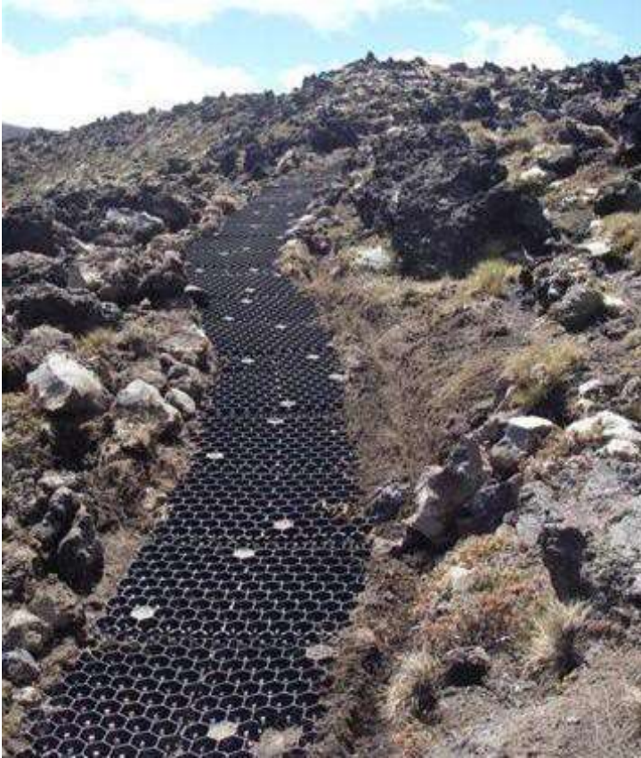
Figure D6: 'Geomat' surface stabilisers (prior to having aggregate placed on top), Tongariro National Park (Photo: John Bradley)
