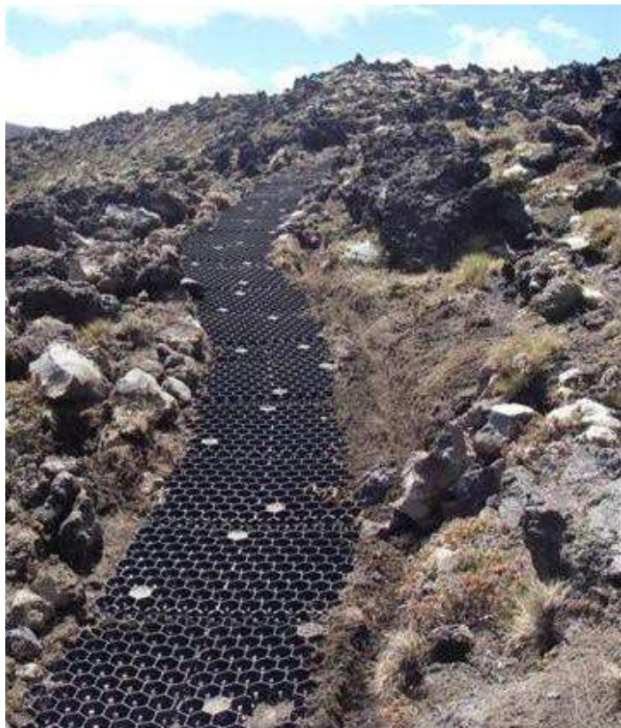
Figure C6: ‘Geomat’ surface stabilisers (prior to having aggregate placed on top), Tongariro National Park (Photo: John Bradley)
