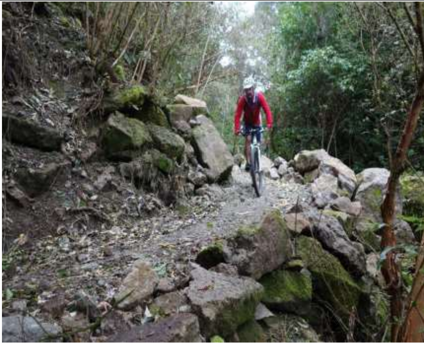
Figure D7: Rock armoured path – Nichols Creek Track, Dunedin (Photo: Kennett Brothers)
