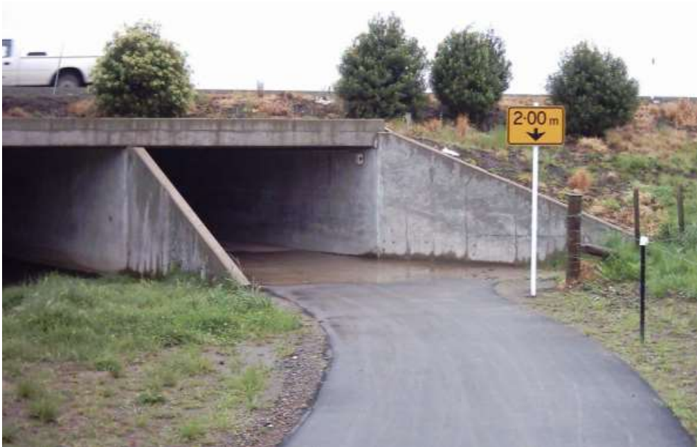
Figure D2: Warning sign for a low underpass, Nelson
