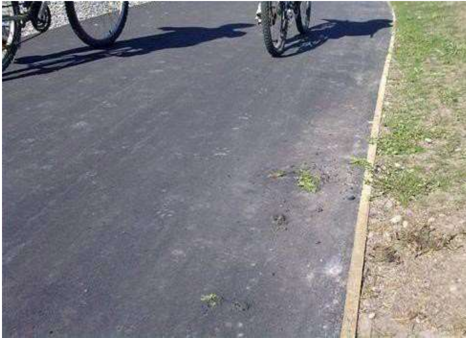
Figure 76: Vegetation growing through new asphaltic concrete path; good construction specifications and contract supervision are required
