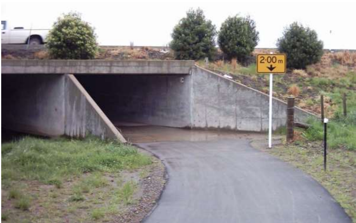
Figure C2: Warning sign for a low underpass, Nelson
