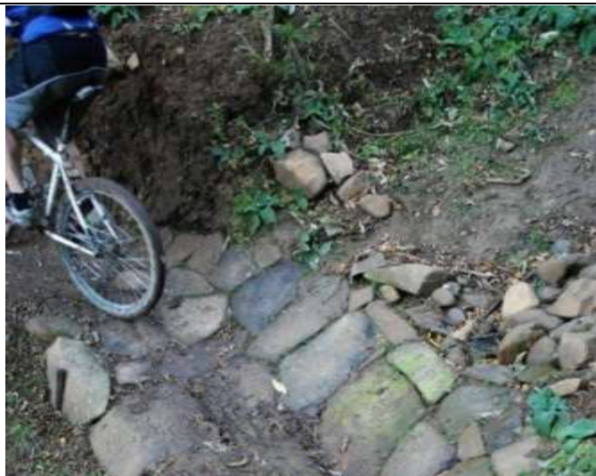
Figure B6: Rock armoured path – Nichols Creek Track, Dunedin (Photo: Kennett Brothers)
