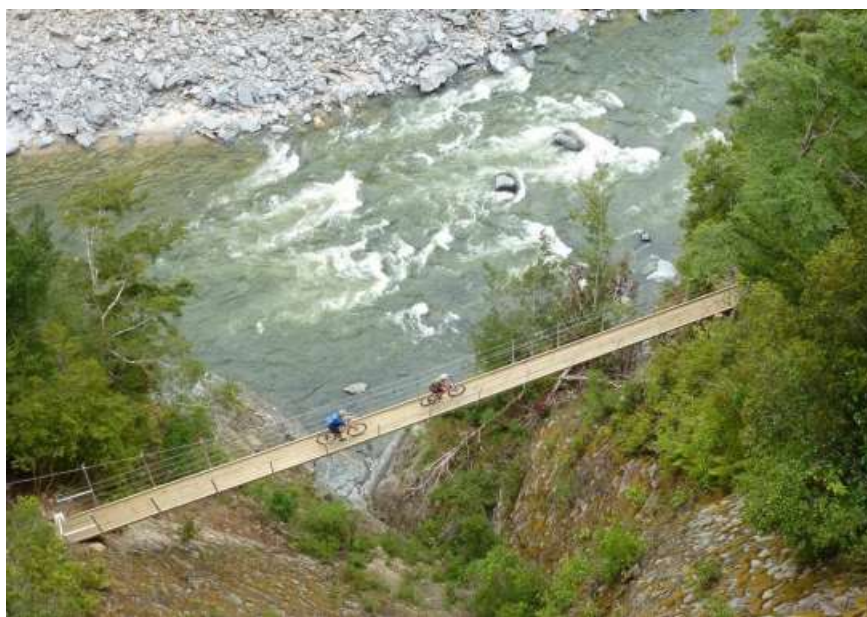
Figure E16: Suspension bridge on the Old Ghost Road (Photo: Jonathan Kennett)
