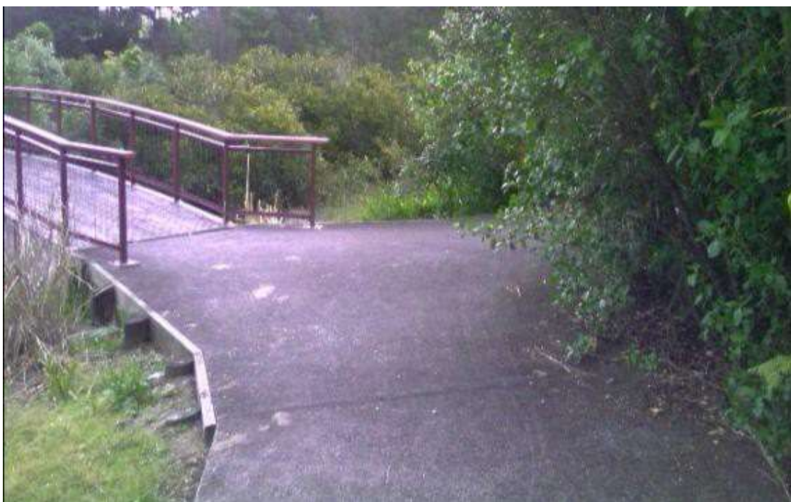
Figure 31: Poor inter-visibility at path intersection – Auckland
