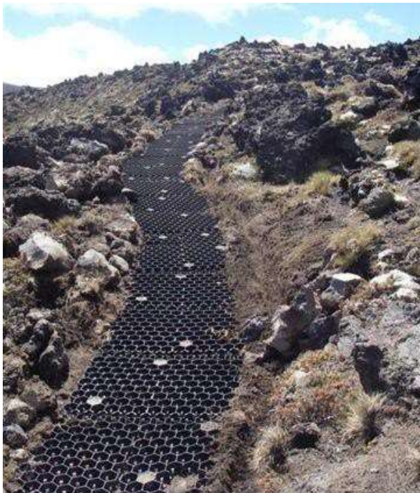
Figure B5: 'Geomat' surface stabilisers (prior to having aggregate placed on top), Tongariro National Park (Photo: John Bradley)
