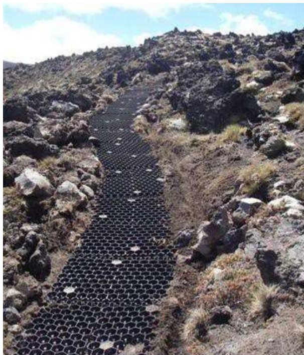
Figure E6: 'Geomat' surface stabilisers (prior to having aggregate placed on top), Tongariro National Park (Photo: John Bradley)
