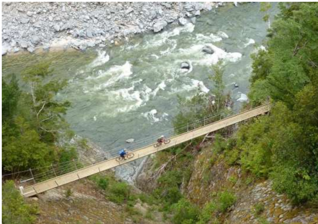
Figure D16: Suspension bridge on the Old Ghost Road (Photo: Jonathan Kennett)
