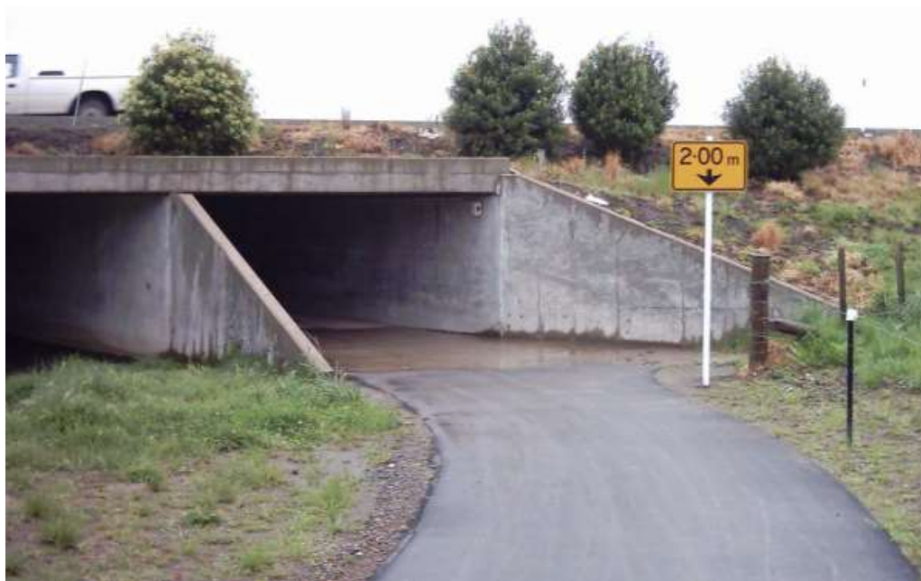
Figure B2: Warning sign for a low underpass, Nelson
