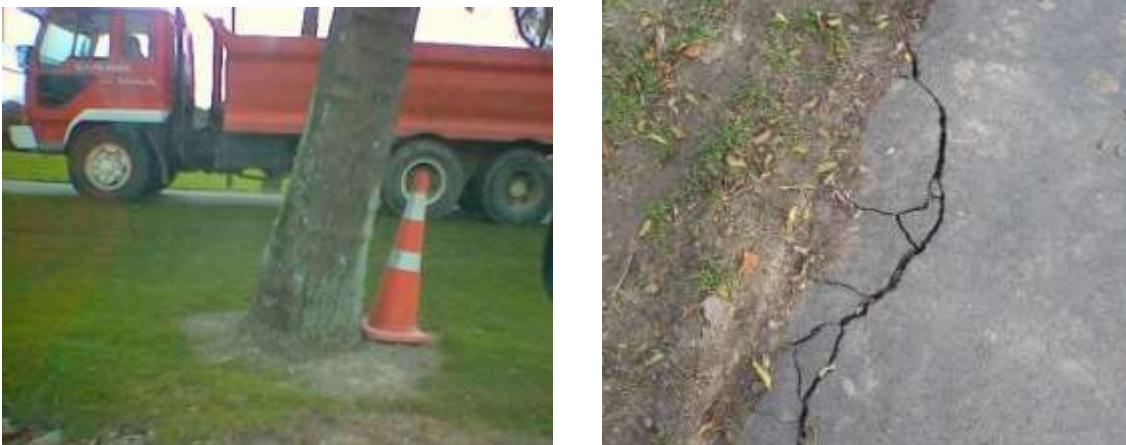
Figure A8: Heavy truck causing edge break on new pathway during construction
