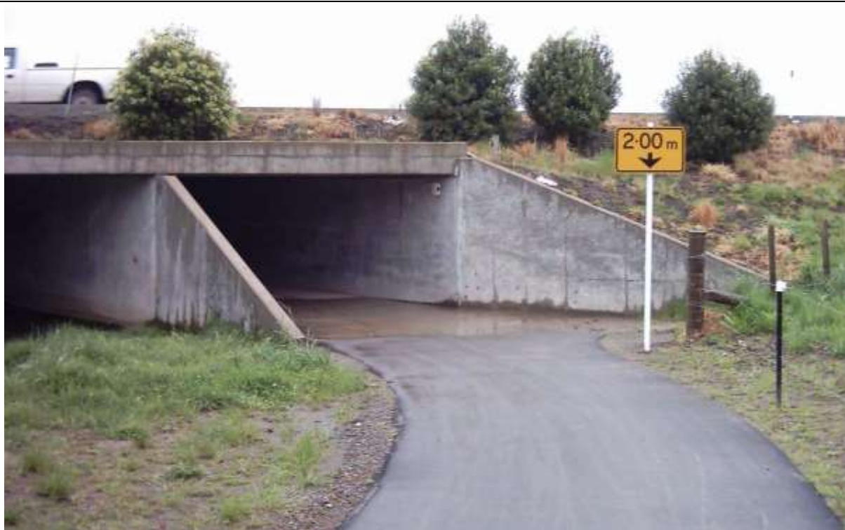
Figure E2: Warning sign for a low underpass, Nelson
